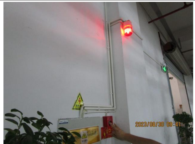
Fire alarm test
