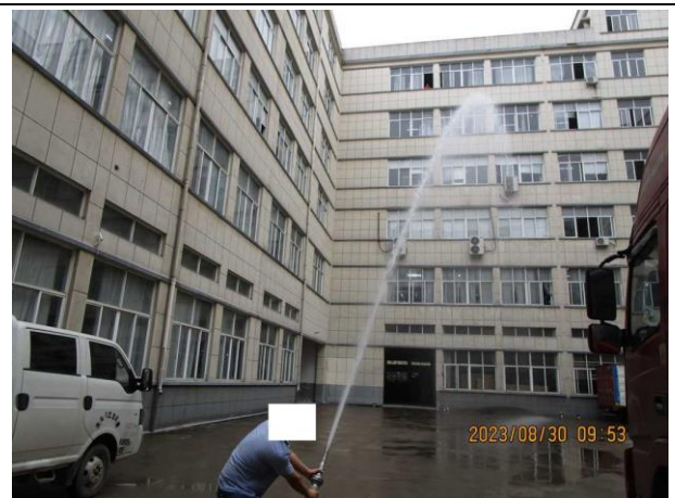
Fire hydrant test
