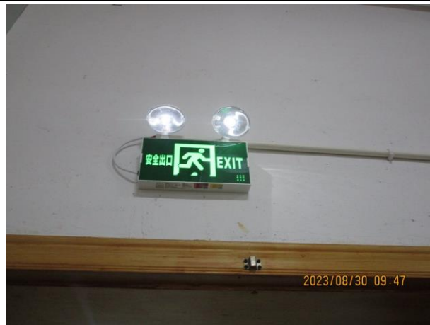
Emergency light test
