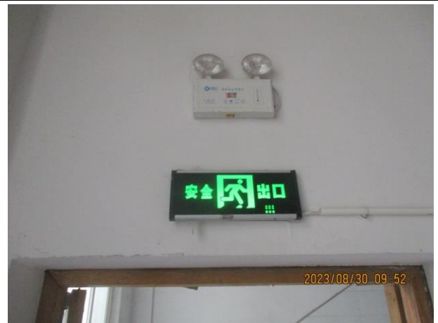
Exit sign and emergency light
