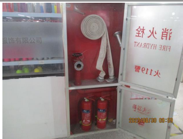
Fire hydrant and Fire extinguisher
